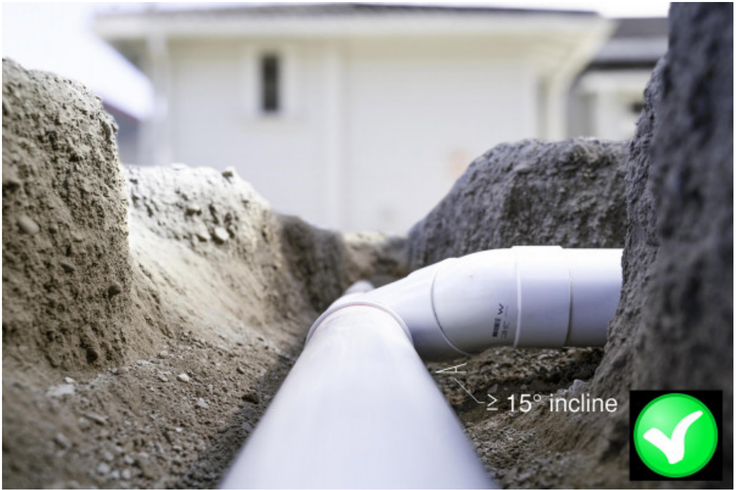
DN100 drain with 45° 'Y' junction installed with a \geq 15^\circ incline above horizontal.
