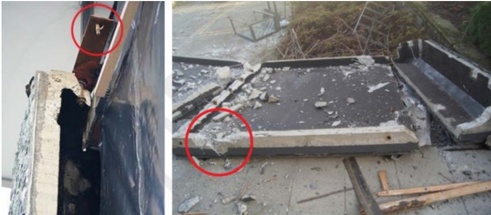
Figure 1: Precast panel connection failures during a Canterbury earthquake. Source: NHRP. The failed connections are circled.
