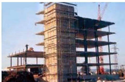
Figure 1: Example of building with poor structural layout of bracing elements
