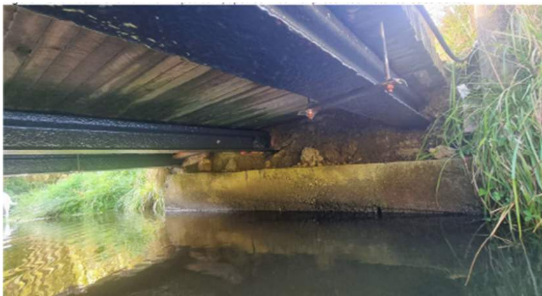
Figure 3: Photo of the bridge and true right abutment. The treated rail beams, and stainless-steel rods and plates tying down the deck, are also shown.
