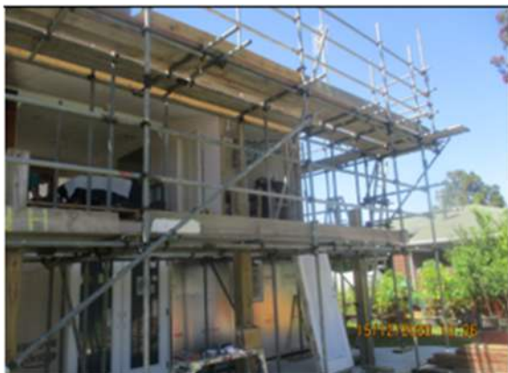
Figure 8: Photo showing the first-floor wall removed and new timber beam/lintel in place (taken 15 December 2020).
