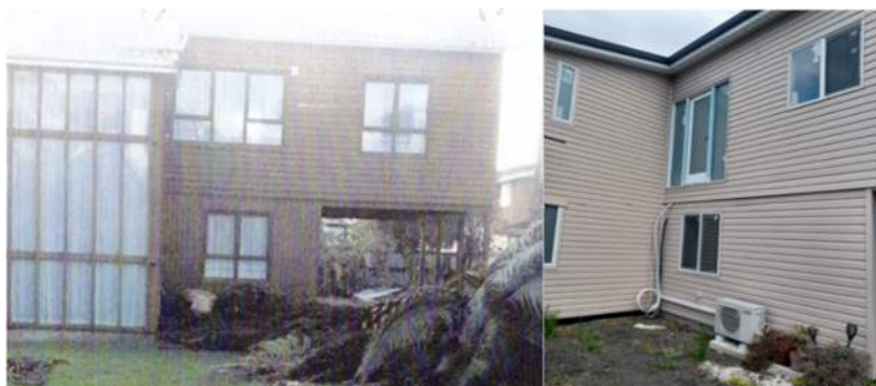
Figure 5: Left - photo showing the former cladding on the south elevation, including the former carport and internal stairwell area (dated 24 July 2018). Right - photo of the south elevation, showing new cladding installed (dated 13 December 2024).
