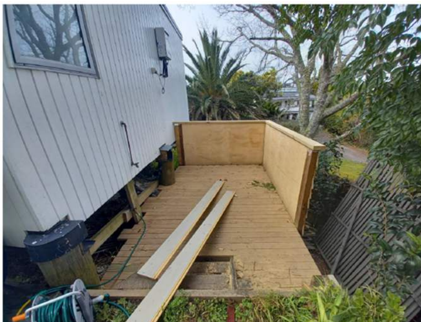
Figure 1: Photograph of the deck and barrier, taken by the authority on 2 September 2025.
