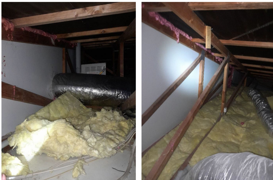
Figure 3: Photos from the 2024 inspection of ducting and fire separations in the ceiling space.
