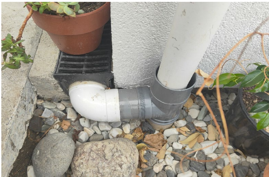
Figure 1: The channel drain
