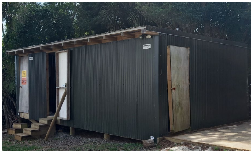
Figure 1: The building the subject of the notice to fix 1
