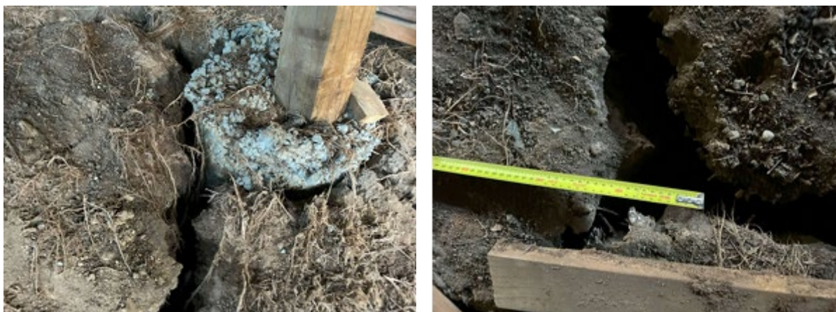
Figure 3: Ground cracking under the dwelling around piles
