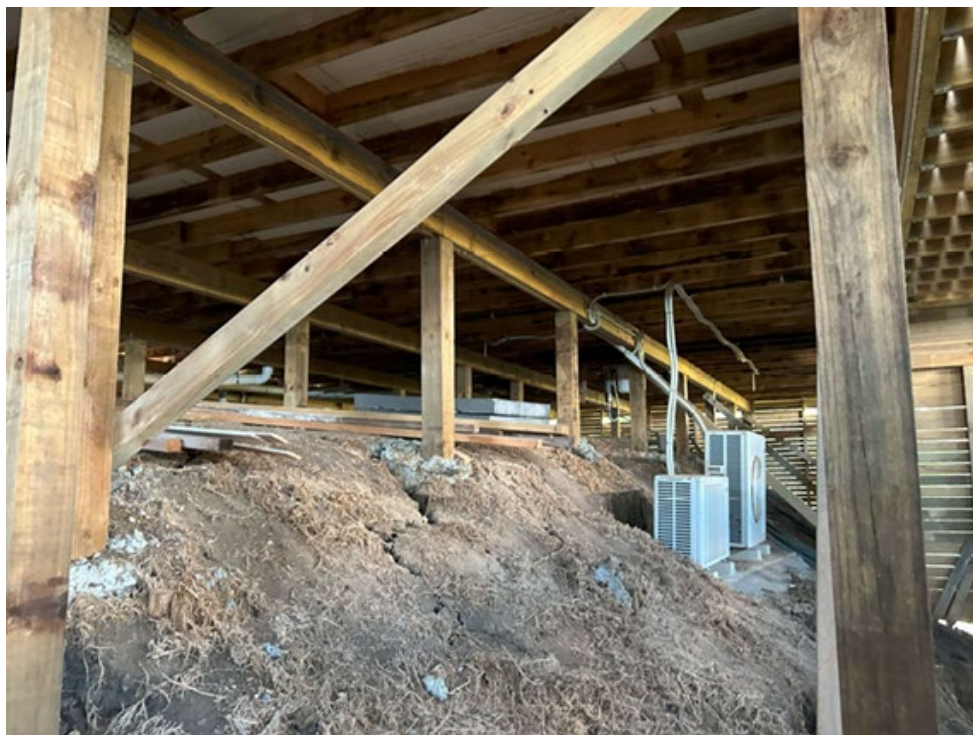
Cover Image: Dwelling sub-floor with piles, concrete encasement and cracking
