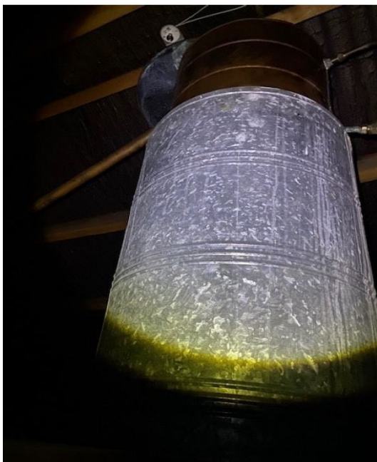
Figure 4: The existing hot water cylinder
