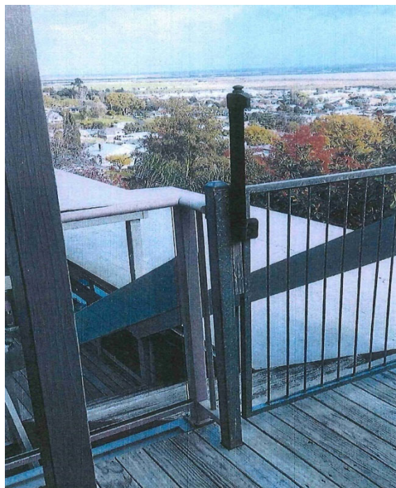
Figure 1: Elements of the pool barrier giving rise to the dispute
