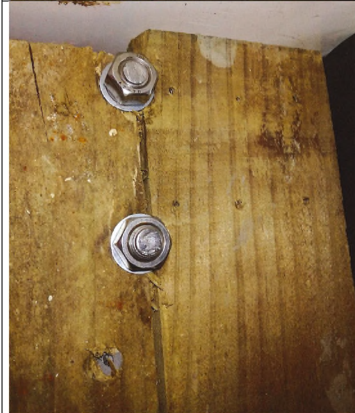
Photograph 5 showing both bolts fixing to the metal angle bracket supporting the SHS above.
