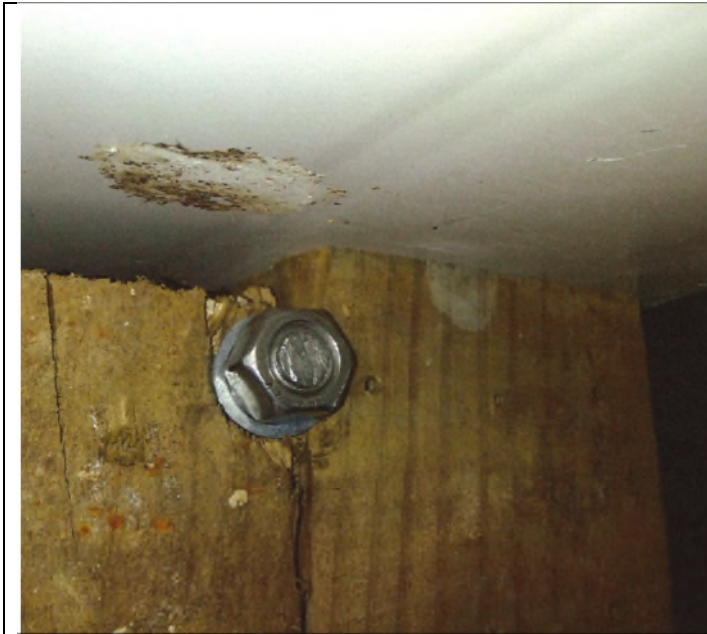
Photograph 4 showing the top bolt fixing to the metal angle bracket supporting the SHS above (the photograph is taken from the other side of the pile from Photograph 3).
