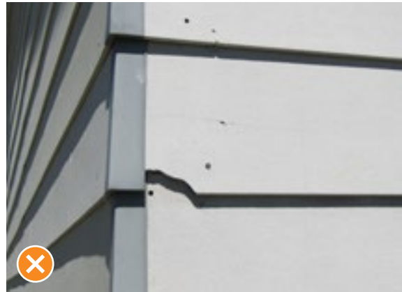
Figure 15 Damaged fibre cement weatherboard.
