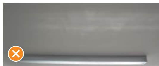
Figure 22 Sheen banding on a finished ceiling that is clearly visible from normal viewing position under non-critical lighting conditions. Source: Winstone Wallboards
