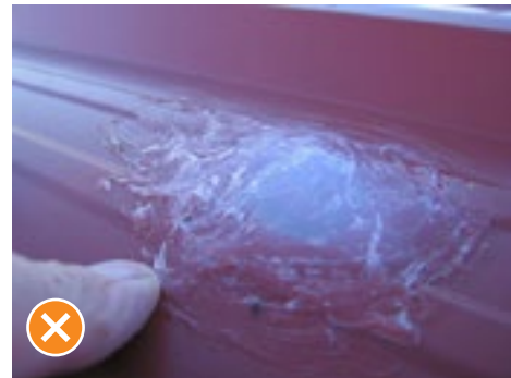
Figure 19 Sealant-filled fixing hole with untidy finish.
