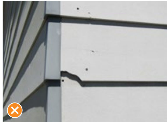
Figure 15 Damaged fibre cement weatherboard.
