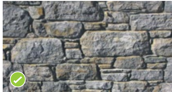
Figure 11 Acceptable stone work – joints are of an even size. Vertical joints are less than 300 mm high, and stones are regularly crossed to form good bonding. Source: NZSMA
