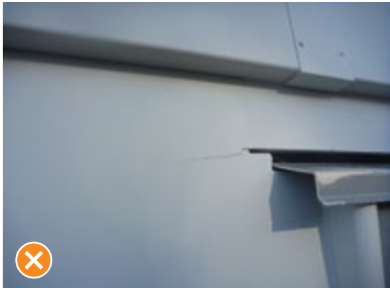
Figure 14 Crack in a fibre cement weatherboard.
