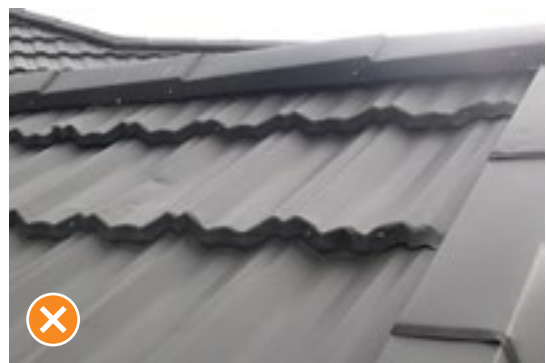
Figure 17 Dented metal tiles.
