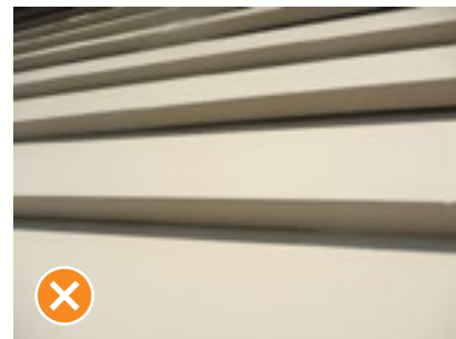
Figure 13 Gap of more than 2 mm between weatherboard laps on a light coloured painted wall.
