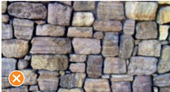
Figure 10 Stones are stacked on top of each other with continual running vertical joints and very little bonding. Source: NZSMA
